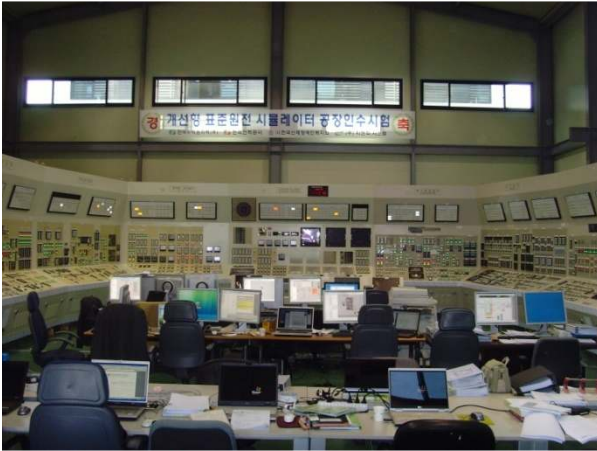
Fig. 1. Overall View of OPR1000 Simulator
