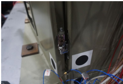
Fig. 3. Structural damage observed at the door hinge of the load center
