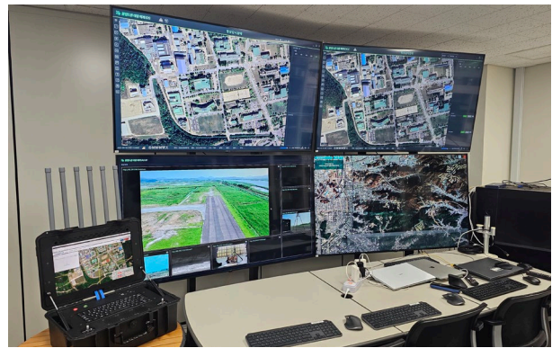
Fig. 4. Picture of ICS operation room
