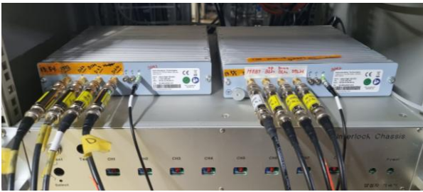
Fig. 3. Installation and operation of LIBERA ADC and EPICS
