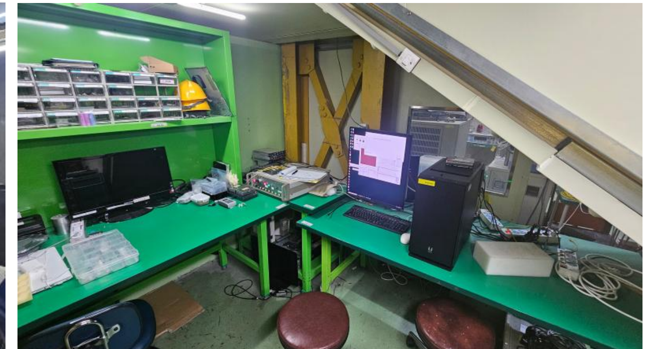
Remote control room
