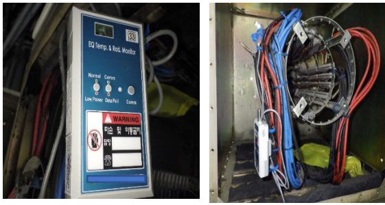
Figure 3. A typical example of installing a temperature monitor.
