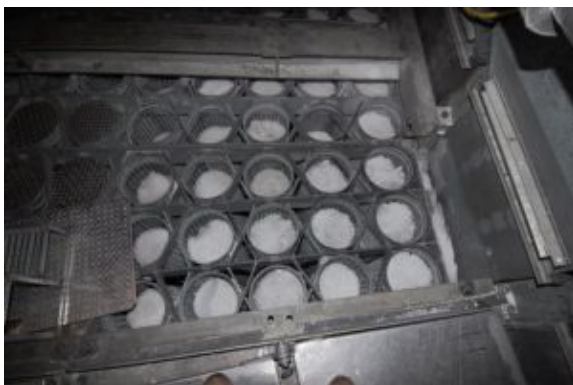
Figure 1. Ice condenser of DC Cook NPP (US)
