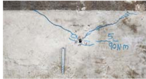
Fig. 4. Concrete breakout failure
