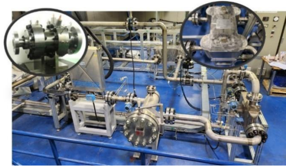
Fig. 1. Photograph of the Helium Supply System (HeSS) facility with the helium circulator and the economizer
