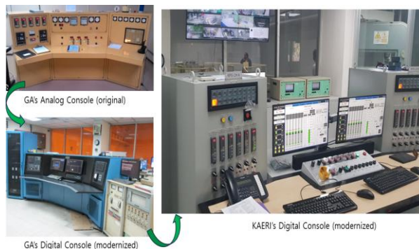
Figure 2. I&C systems refurbishment of Bangladesh 3 MW TRIGA Mark II research reactor
