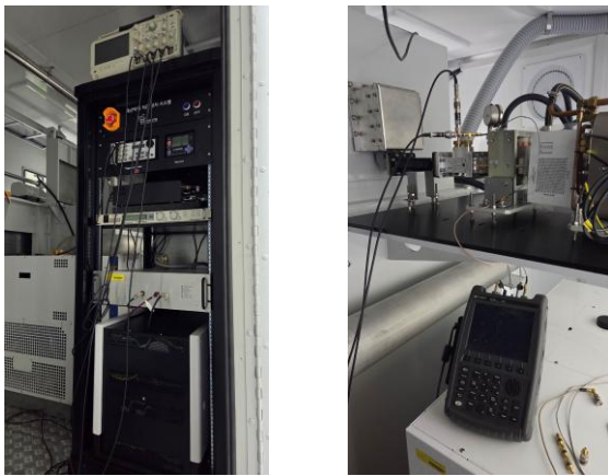
Figure 4. Equipments installed in the vehicle
