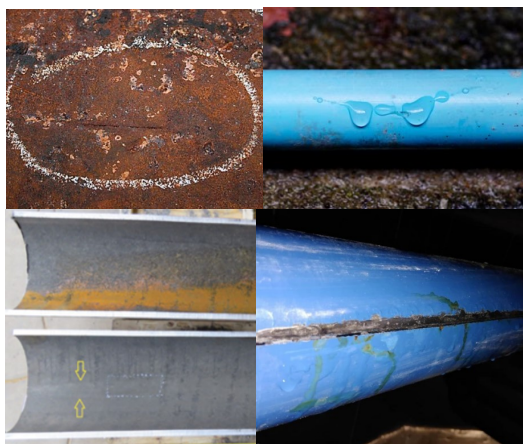
Fig. 1. Various types of pipe damage.
