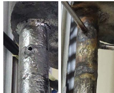
Fig. 3. the broken part by corrosion(left), the repair weld of a broken part, and the heat affected zone(right).
