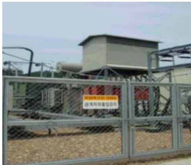
Figure 6. Transformer/rectifier tank, capacitor filter
