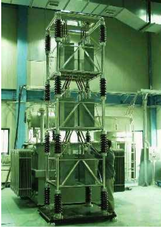
Figure 2. IVR, transformer/rectifier tank, filter
