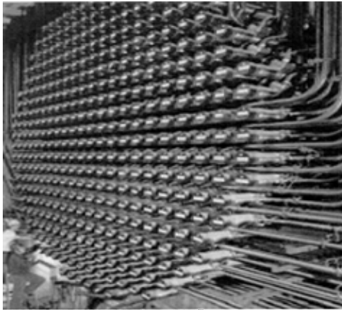
Figure 1. Feeder pipes in PHWR Reactor.
