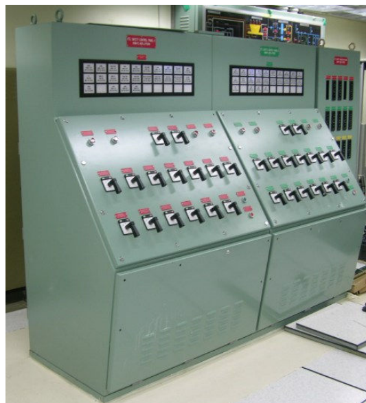
Fig. 3. Picture of FTL safety control panels and FTL indicator panel.
